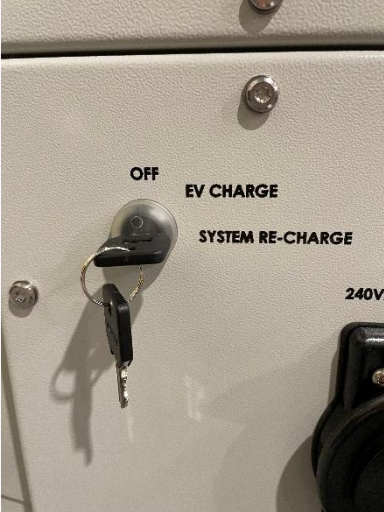
Figure 14—Key Switch in SYSTEM RE-CHARGE position
