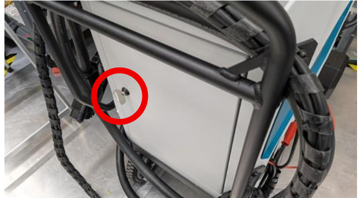
Figure 33: Outdoor Mobile EV Quick Charger front door, closed and locked with door key
