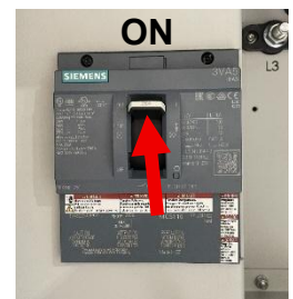
Figure 22—AC Main Switch ON
