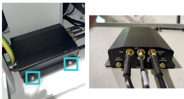
Figure 24—Modem anchored to charger floor with 4 screws and right-side (face view) of installed modem with cables still attached
