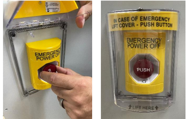
Figure 53 - Reset Emergency Power Off button
