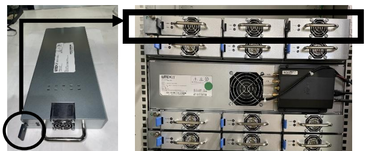
Figure 34 – Inverter modules (black tabs) installed in upper shelf of Inverter Shelf Set | 21
