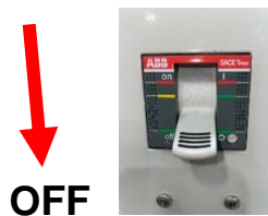
Figure 4—AC main power switch in the OFF position
